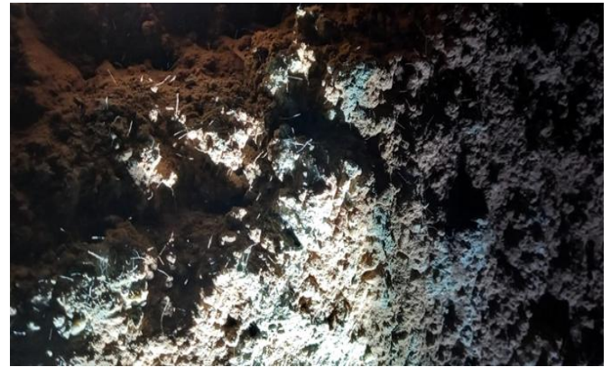
Figure 12. Condition of the fiber-reinforced shotcrete lining in the transition zone ( r = 5-7 m) after blasting of fan-pattern blastholes: localization of crack formation without loss of bond to the rock mass
