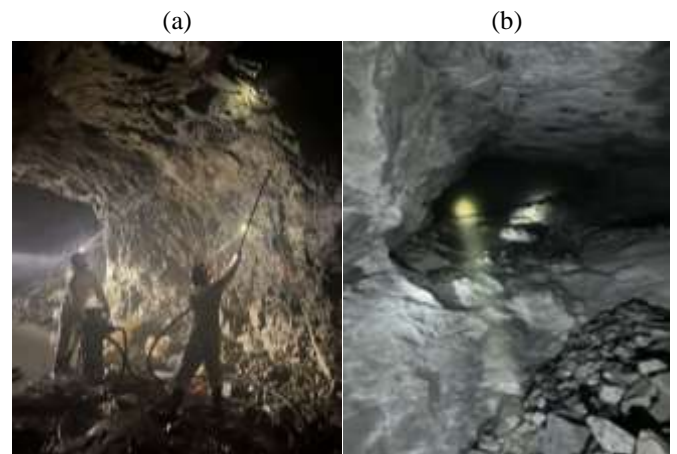
Figure 9. Experimental-industrial tests of breaking thin slope ore bodies in the Akbakai mine using charges with controllable blast characteristics
